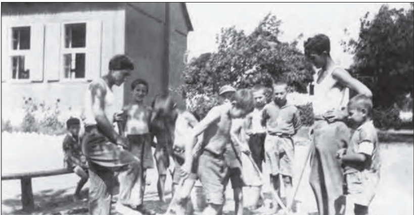
Paving the paths between the bungalows at the summer camp. Photographed by Shlomo in 1934.
